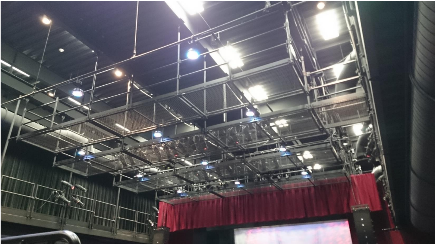
Lighting grid front of house from audience.
