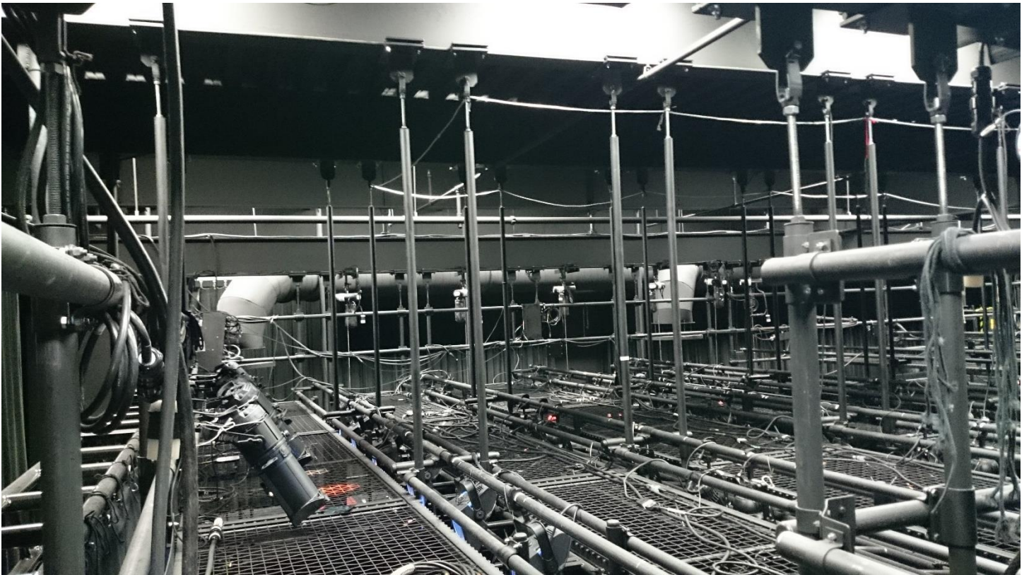
Lighting grid upstage overhead.
